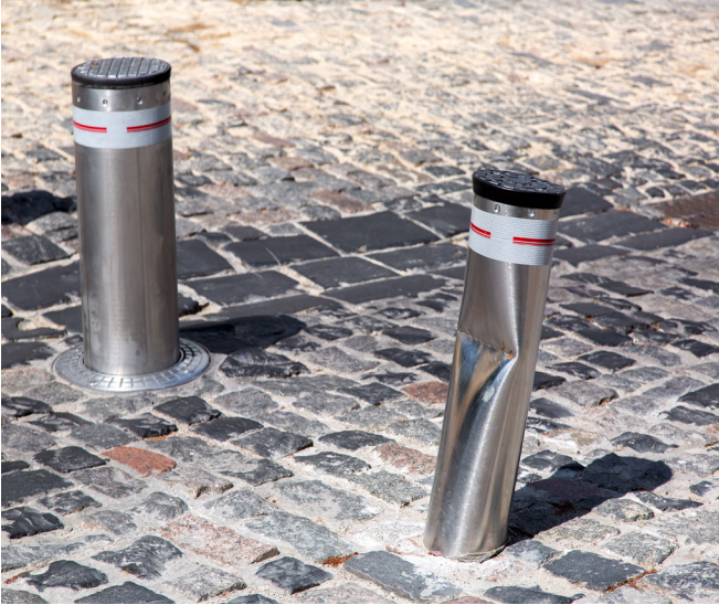
Damage from a standard vehicle
